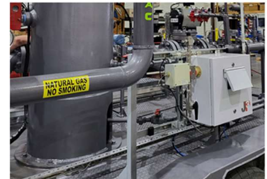
Frac Trailer Mounted System
